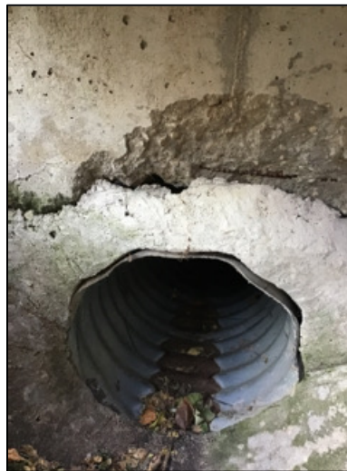
Figure 14. Structure Condition: Poor.
