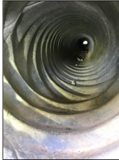
Figure 18. Pipe Condition: Good. Pipe shows some signs of aging or very minor defects
