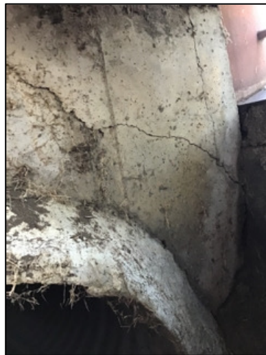
Figure 13. Structure Condition: Fair.
