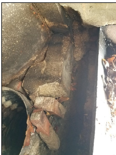
Figure 15. Structure Condition: Failed.
