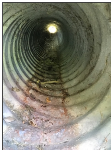
Figure 20. Pipe Condition: Poor. Corrosion and minor holes along invert of pipe
