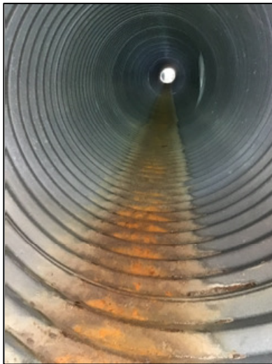
Figure 19. Pipe Condition: Fair. Minor to moderate corrosion along invert of pipe.
