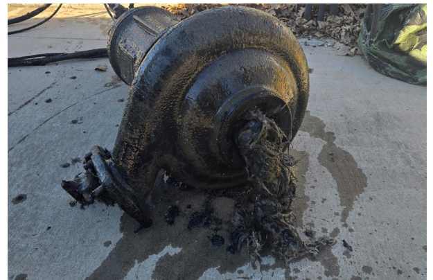
A clogged pump from one of our lift stations
