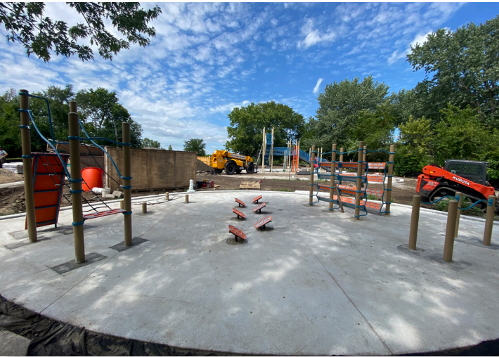
New equipment is installed at Glendell Acres Park. Look for a ribbon cutting this fall!
